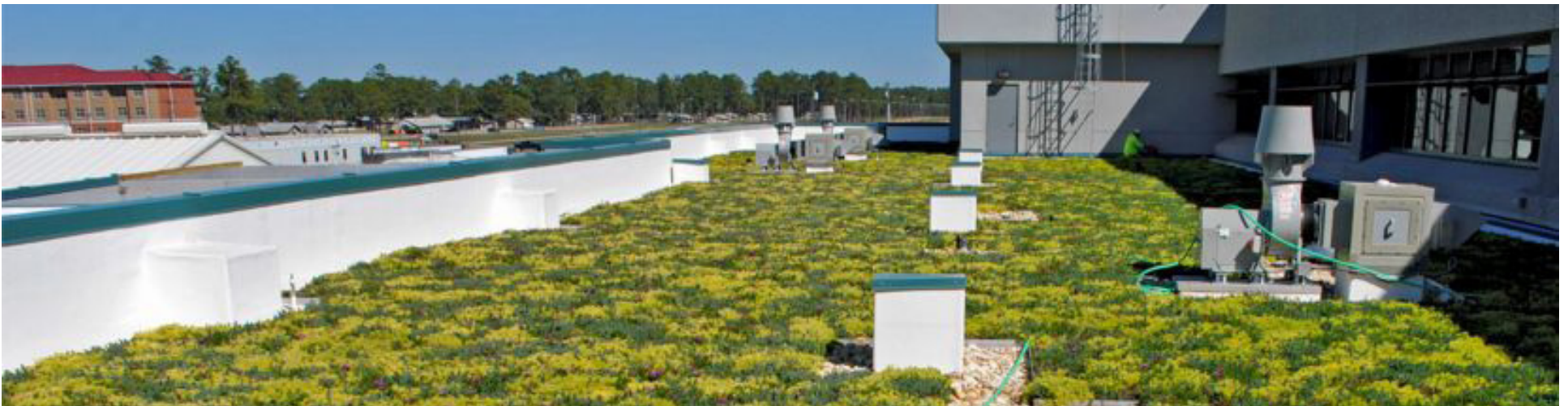
Example of a green roof at the Federal Army Hospital at Fort Stewart, GA
