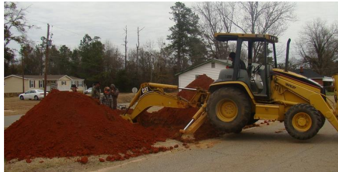
Even seemingly simple repairs can be costly if happening at the wrong time or place. The City of Jeffersonville would spend nearly $50,000 to repair this broken water main under U.S. 80.
