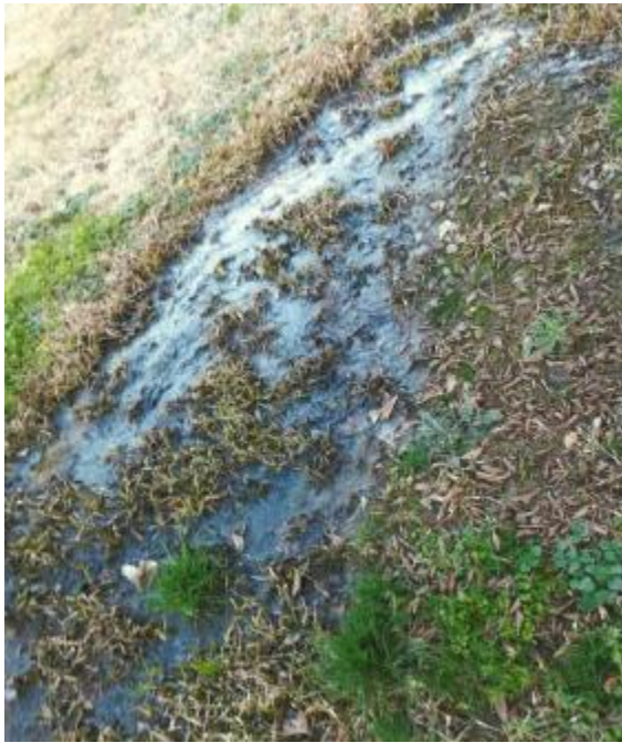
In southwestern Jones County, old septic systems were causing leakage of sewage into homes and yards. The county is currently fixing the problem with new sewer lines.
