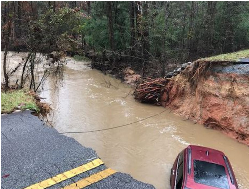
Above: Erosion from flooding washes out Rocker Road, leaving one woman injured. Source: WRDW web article published Jan. 13, 2020
