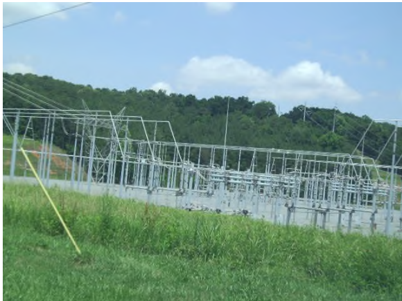
Power substation east of site
